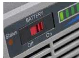
An extra control panel for the battery: ON/OFF switch, LED display showing the battery charging state
